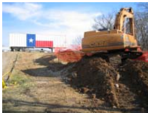
DANGER: Do not fall into this hole!
