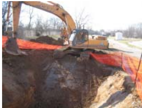
Big sewer leak
